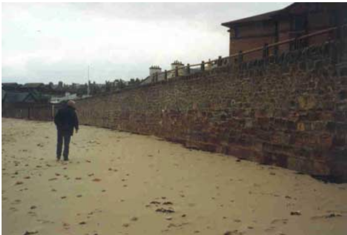
Plate 9.40 Defence No 51 Dunbar East Beach, Masonry wall at new flat development
