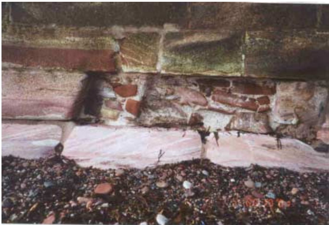
Plate 9.36 Defence No 47 Dunbar East Beach, Scoured hole at base of wall
