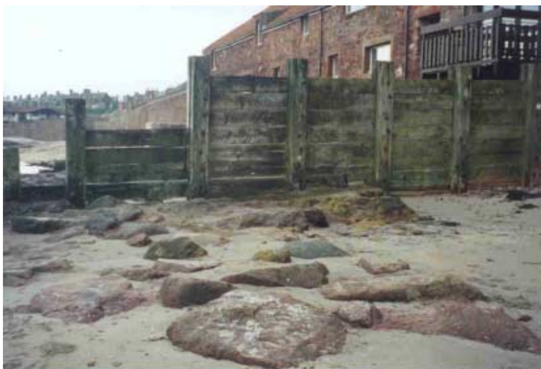
Plate 9.38 Defence No 48 Dilapidated Groyne (Dunbar East Beach)
