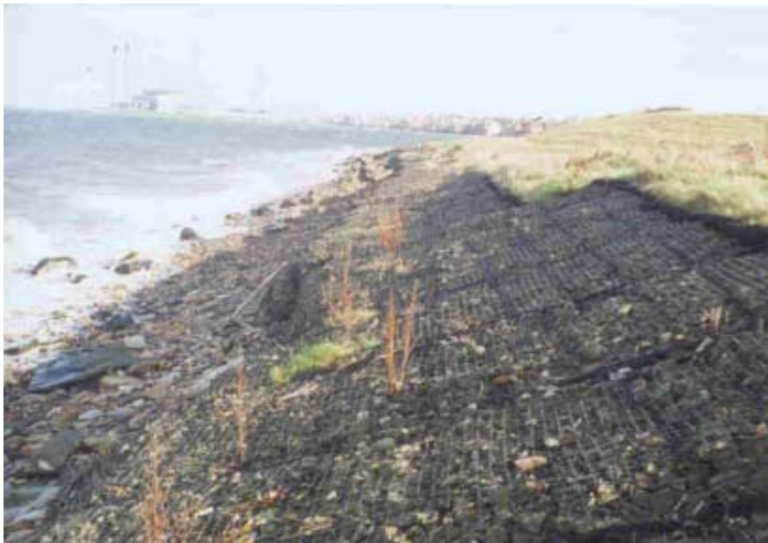
Plate 9.6 Defence No 10 Gabions at the Cast (Good Condition)
