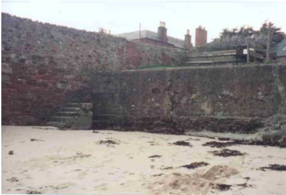
Plate 9.39 Defence No 51 Dunbar East Beach, Garden walls in need of repair
