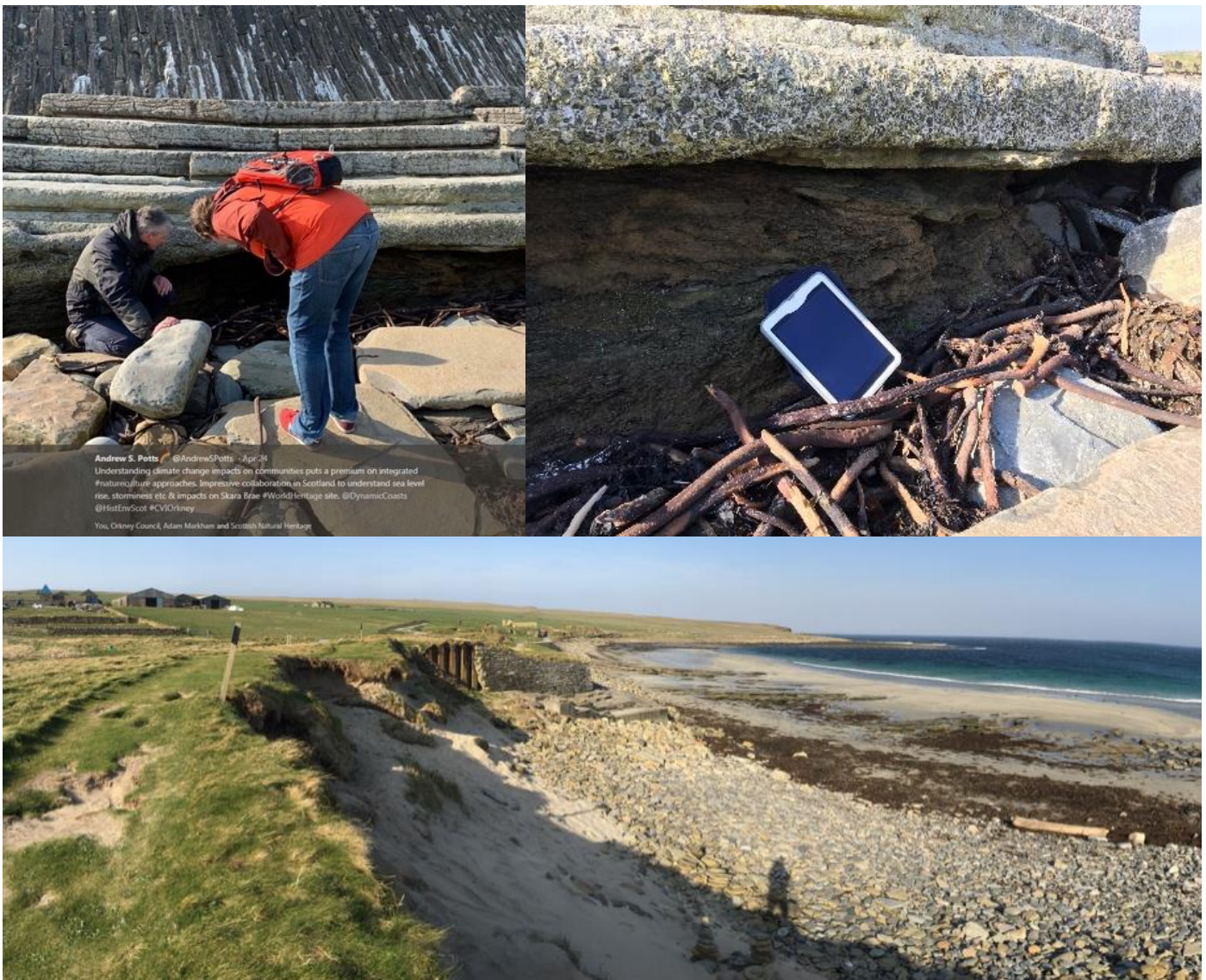
Figure 18 Skara Brae sea wall showing latest phase of undermining of toe concrete to expose friable bedrock beneath. Bottom scene shows seawall end flanking and erosional bight resulting from \sim 0.4 m/yr retreat of Vegetation Edge, which now lies 20 m landward from the seawall.
